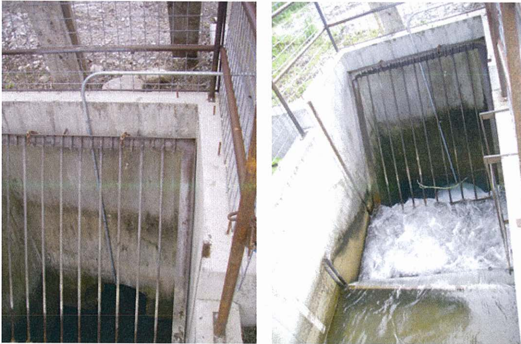
Figure 9 – Inlet conditions at the Upper Diversion the Middle Ditch at no flow (left) and low flow (right).
