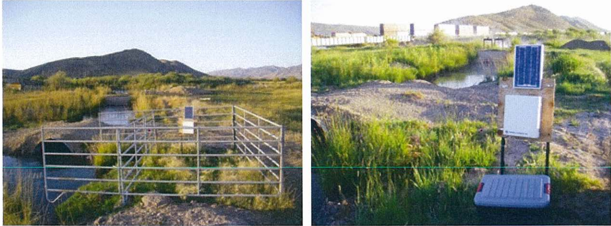
Figure 6 – Installation of DFM systems on Nuffer Diversion. Right hand picture depicts the Unidata DFM deployment, enclosure and power supply are located behind fencing for protection from cattle, squash pipe is located in stream adjacent to DFM system, and the diversion works can be seen in background approximately 100 feet upstream of the squash pipe. The left hand picture is a close up of the Unidata DFM system, note the weather proof container at the base of the fence posts where the MACE DFM system was temporarily housed.
